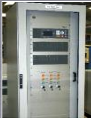
Fire and Gas detection System Control Panel CS400
