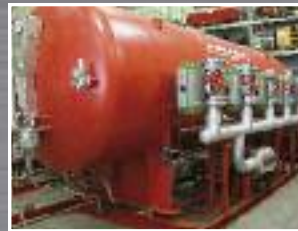
Cryogenic Tank - CO 2 Low Pressure Fire fighting System
