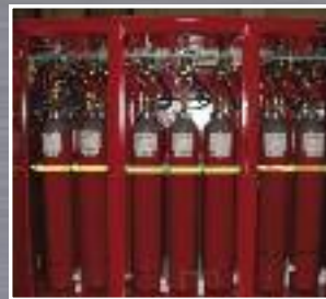
CO 2 High Pressure Fire Fighting Systems
